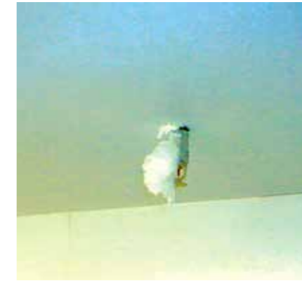
▲ Figure 5: Photograph of dry sprinkler not properly sealed around the sprinkler penetration causing external ice build-up. This condition should be readily visible during an inspection of the sprinkler system.
